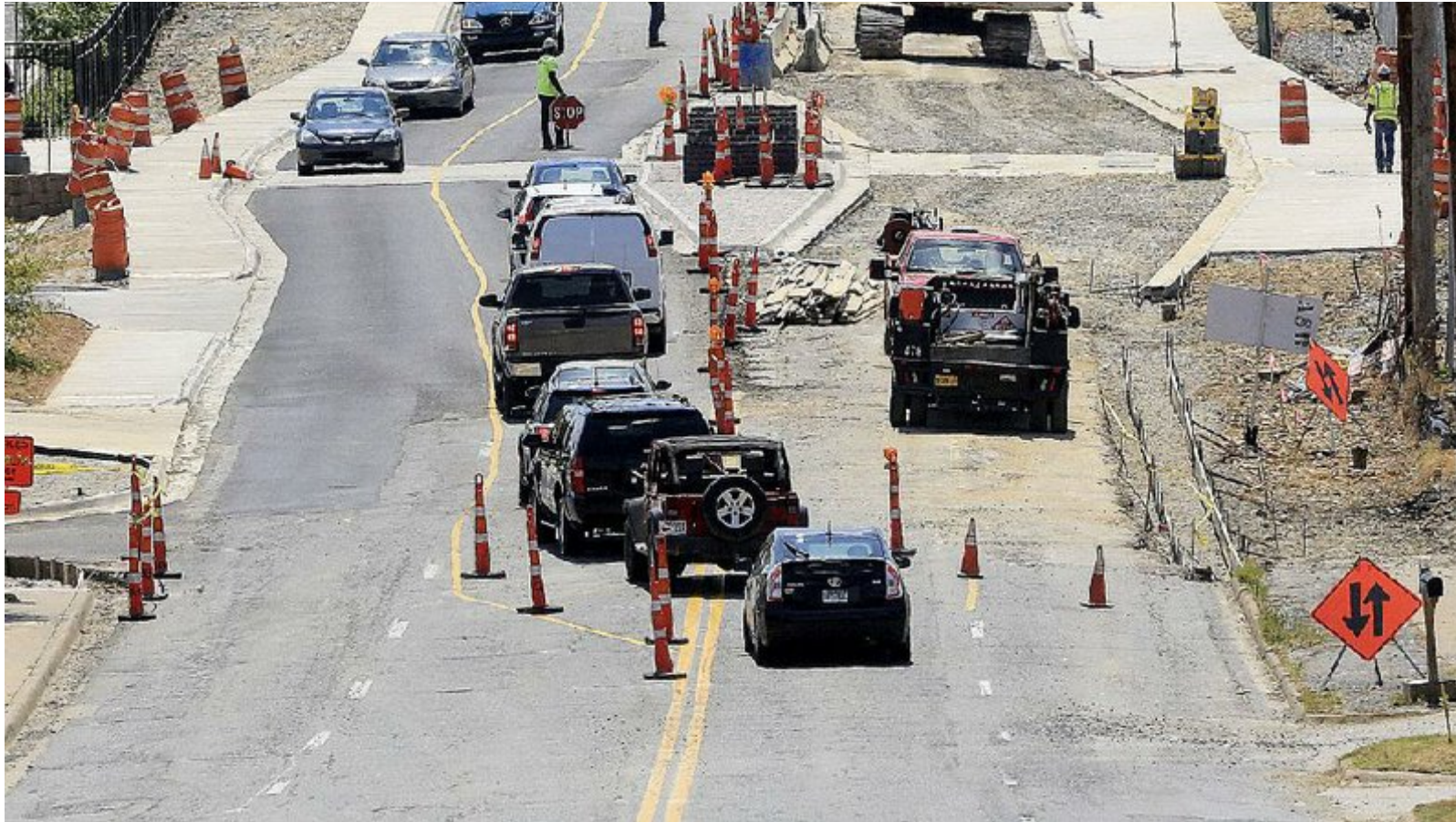
Work continues Friday on a new crosswalk on Main Street near North Little Rock High School. Students will park in a new lot across from the school and will use the crosswalk when classes start Monday. - Photo by Staton Breidenthal
